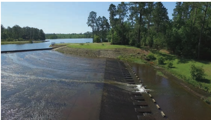
Lake, dam, and spillway built by the CCC at Little River State Park
