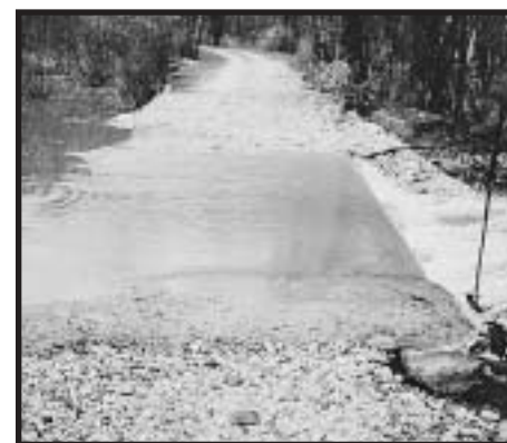
Top left: Insufficient fill material over the top of the pipe contributed to this failure. Top right: This example of good vegetative cover will protect the side slopes of the road and decrease the amount of sediment reaching the stream. Bottom left: A geo-web ford, when properly installed can be a good alternative to a culvert in the right situation. Bottom right: Low-water bridge at flood stage.
