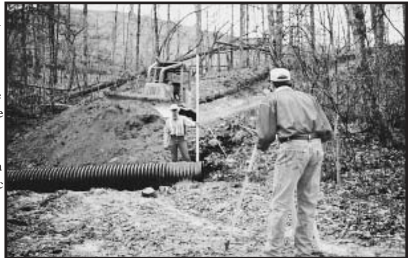
Installing a pipe at the correct elevation and slope, and using good fill material contributes to long-term cost effectiveness.
