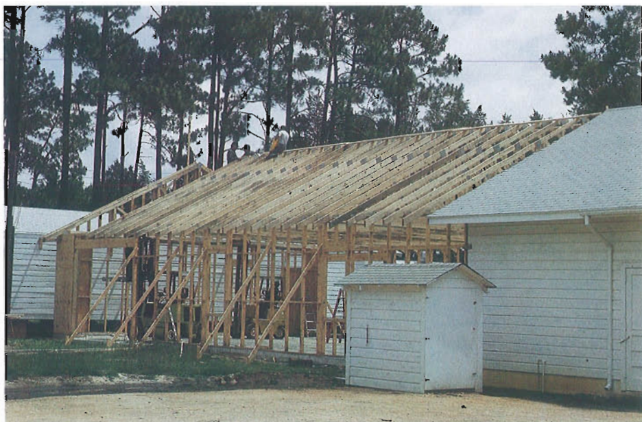
At Hauss Nursery, located near Atmore, an extension to the packing shed was recently completed by nursery personnel.
