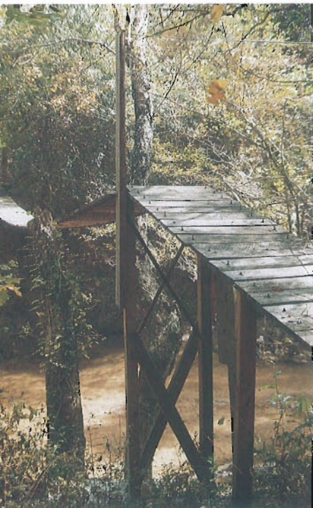
This cable bridge above the creek is one of two found on the Harrison TREASURE Forest.
