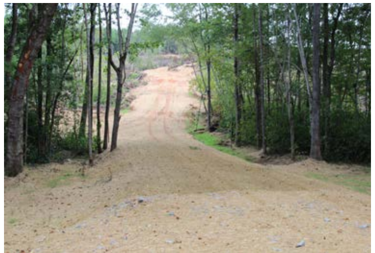
Steep road approaches can present erosion control challenges that can be minimized by the installation of multiple water bars and by eliminating exposed soil through planting grass seed.
