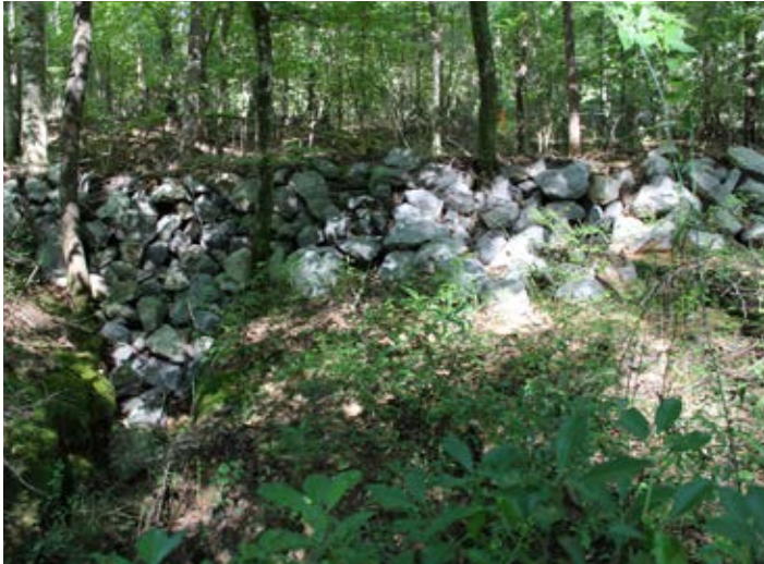
Simple rock check dams such as this one in Tuscaloosa County have captured over 1,000 tons of sediment from dirt roads and are easy to install.
