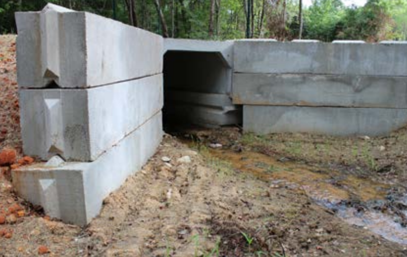
This modified stream crossing structure was designed by Westervelt staff to allow heavy equipment access to timber tracts while also maintaining the integrity of the stream.
