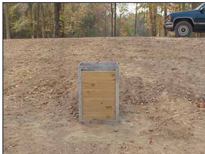
This photo shows a flashboard riser water control structure that has been placed in a newly-constructed levee.
