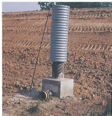
Riser pipe with sleeve for deep water release, valve, and concrete counterbalance.
