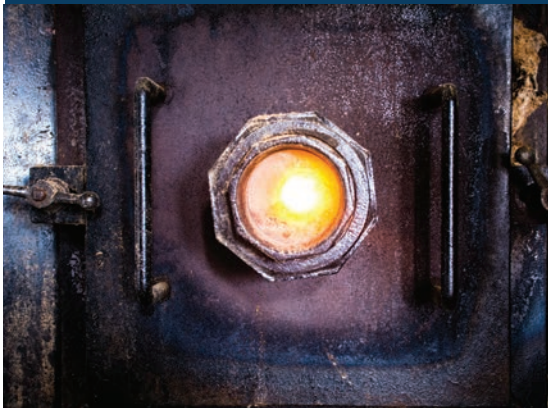
A wood-fired boiler converts sawdust and shavings into 60,000 lbs of steam per hour.
