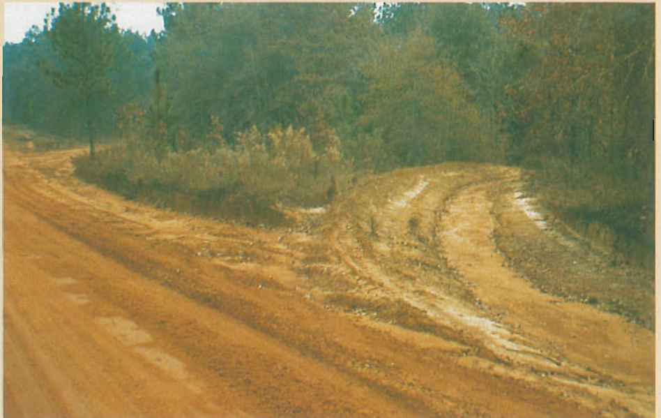
A turnout is used to divert water away from a road or ditch.
